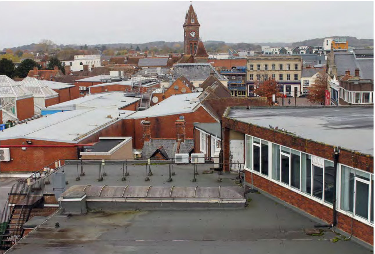
Plate 7: Roof of The Catherine Wheel (OA 40) surrounded by Kennet Centre development, looking north
